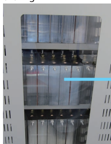
Battery packs undergoing trialing
