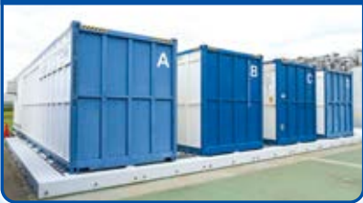
Redox Flow Battery
