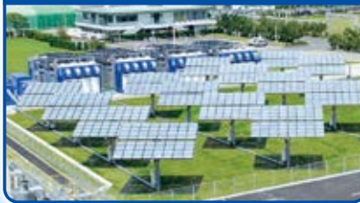
Concentrator Photovoltaic (CPV) System
