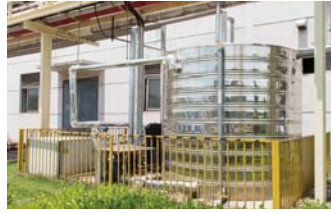
Use of waste heat from sintering furnaces for heating shower water
