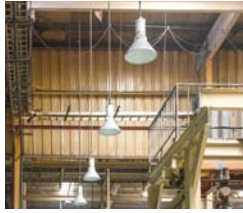
Introduction of LED lights in the plant
