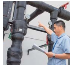
Adjustment of the pressure of cooling water
