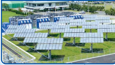
Concentrator Photovoltaic (CPV) System
