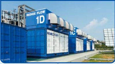
Redox Flow Battery
