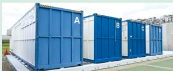
Container type redox flow batteries
