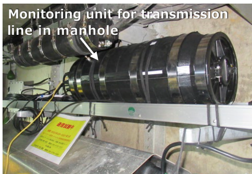
Photo 3. Monitoring unit for transmission line in manhole
