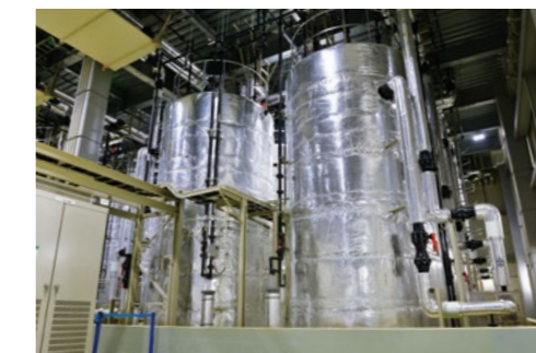
Electrolyte tanks in the building
