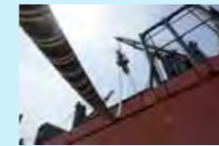
High-voltage submarine cables P.17
