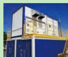
Redox flow batteries
